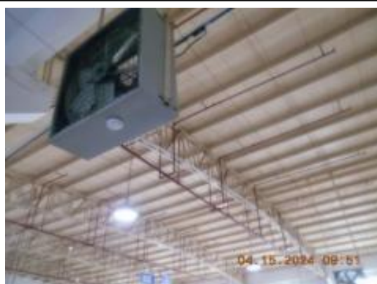
Smoking detector and Fire sprinkler.JPG
