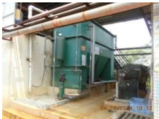
Waste water treatment facility.JPG
