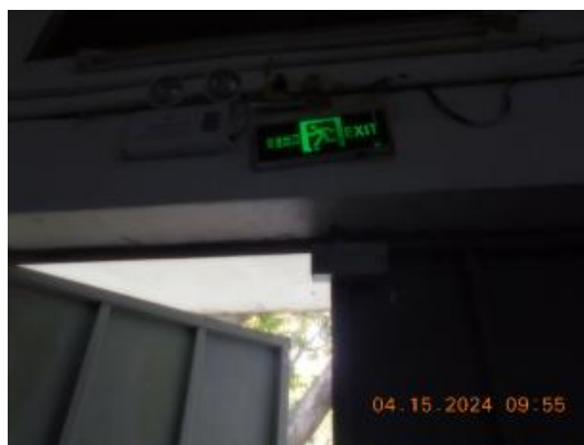
Exit sign and emergency light.JPG
